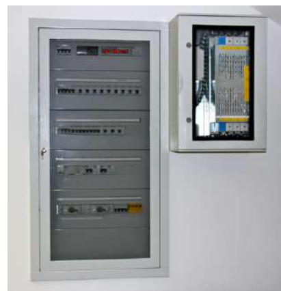
Data Center Protection realised with an ILF 4P 250, installed in the course of refurbishment.
