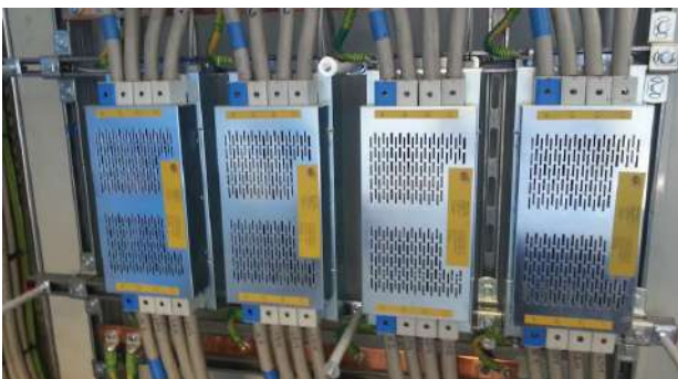
Example of protection for an existing large-sized power distribution panel with ILF 4P 400 surge arrester.
