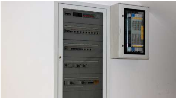
Example of protection for an existing medium-sized power distribution panel with ILF 4P 250 surge arrester.
