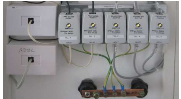
Example of protection for telephony and transmission with S ADLS surge arrester.
