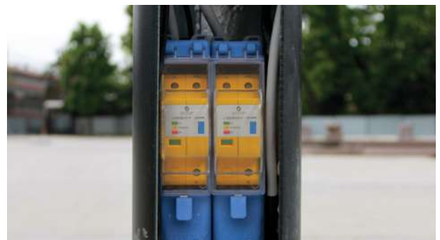
Example of protection in a terminal block for public LED lighting.
